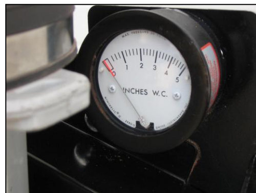
Air Pressure Gage, Which Is Connected to a Port Off of the Accumulator
